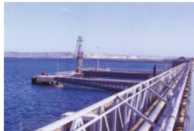
Marine fuel bunker facility at Portland
