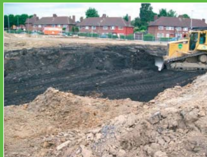
Coal close to the surface being extracted as part of ground works: prevents sterilisation and effective method of remediating unstable ground caused by former coal workings.
