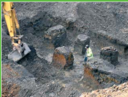
Pillars of coal being extracted as part of ground works: prevents sterilisation and effective method of remediating unstable ground caused by former coal workings.
