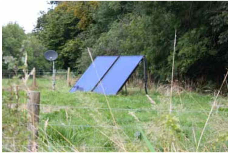
Above: Solar panels at the National Trust's property at Llanerchaeron, near Aberaeron
